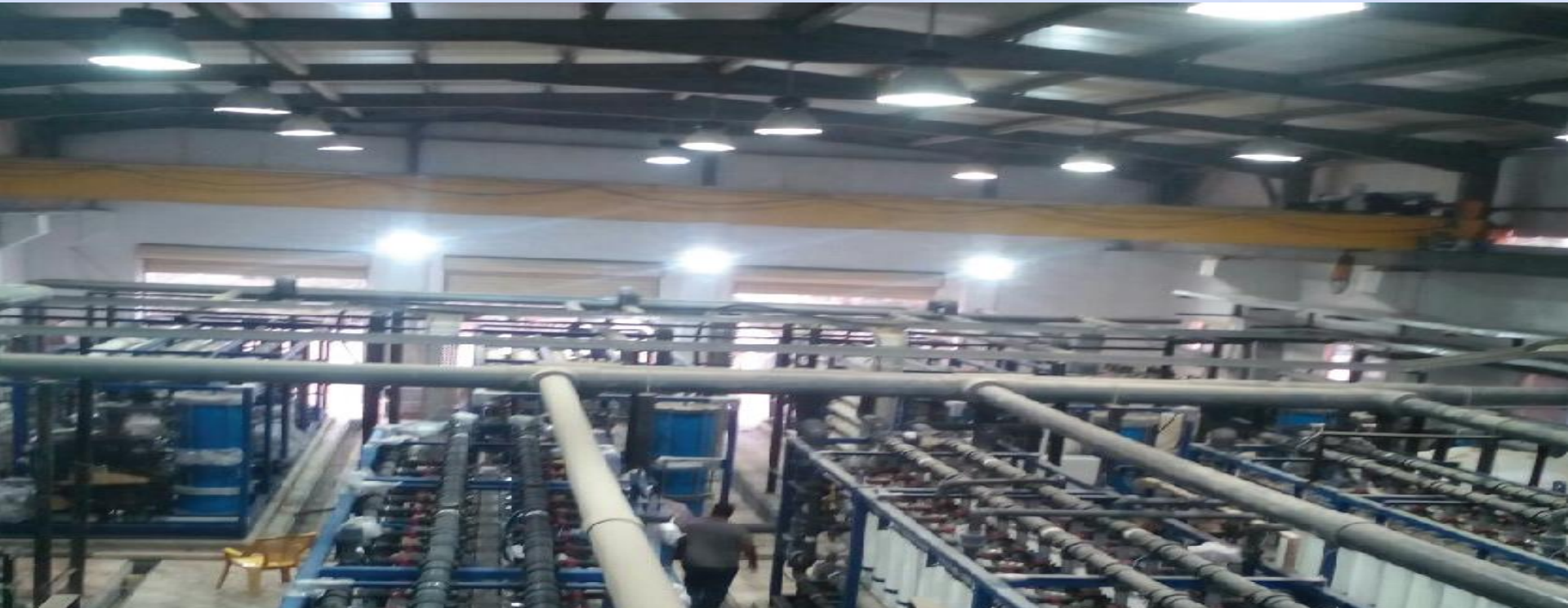
Reverse Osmosis Membranes – Attaqa Power Station
